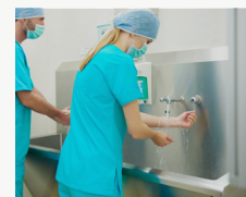
Hospital General Water Systems
